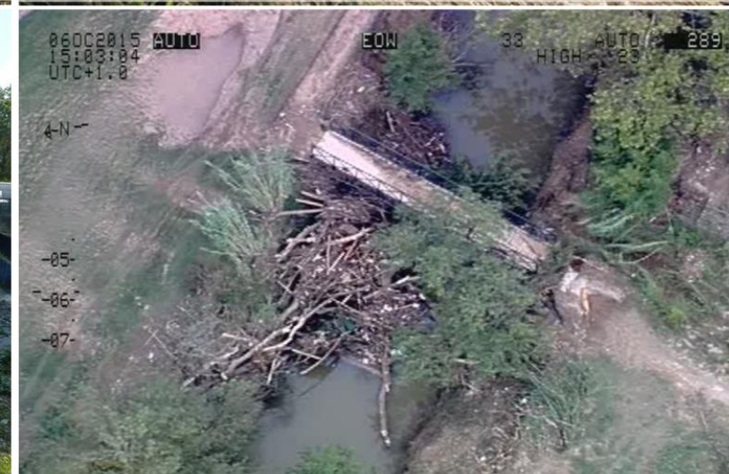
Another bridge clogged by large woods
